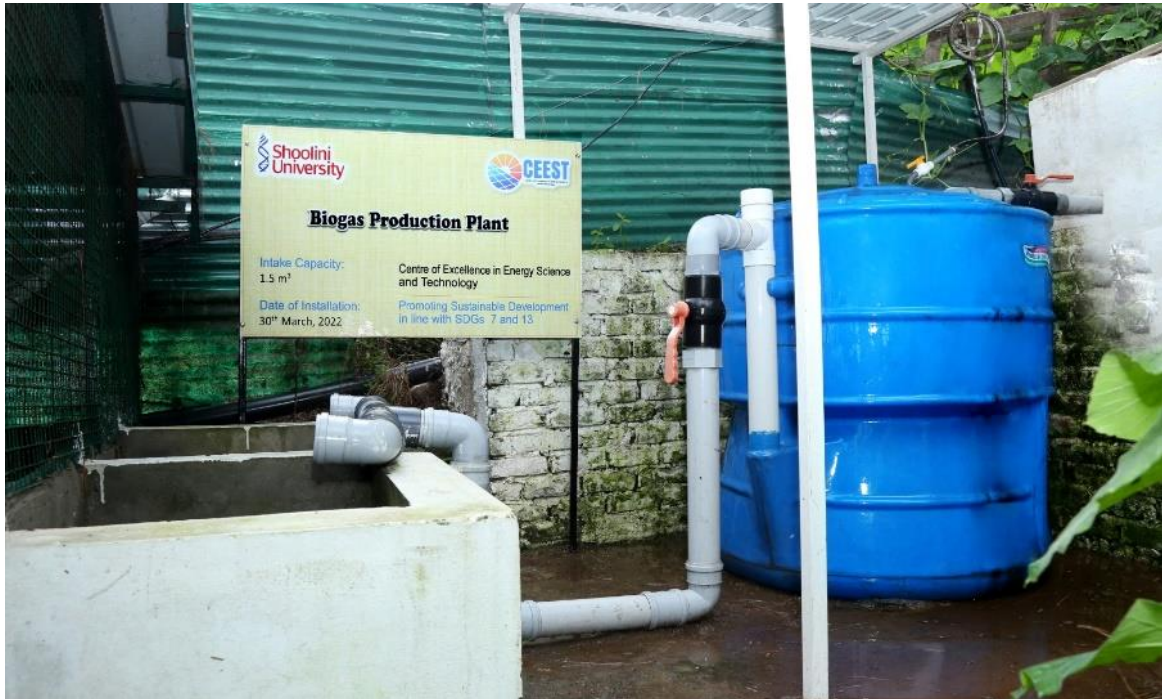
Biogas plant for cooking installed in agriculture farm.
