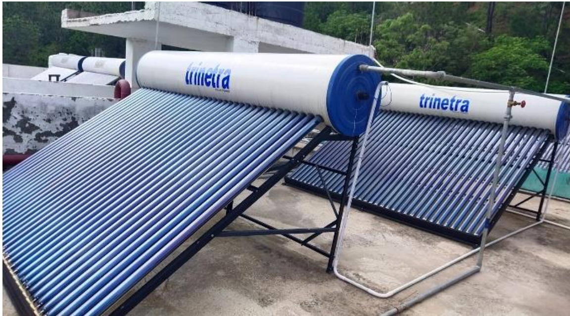
Water heating system on the university campus.
