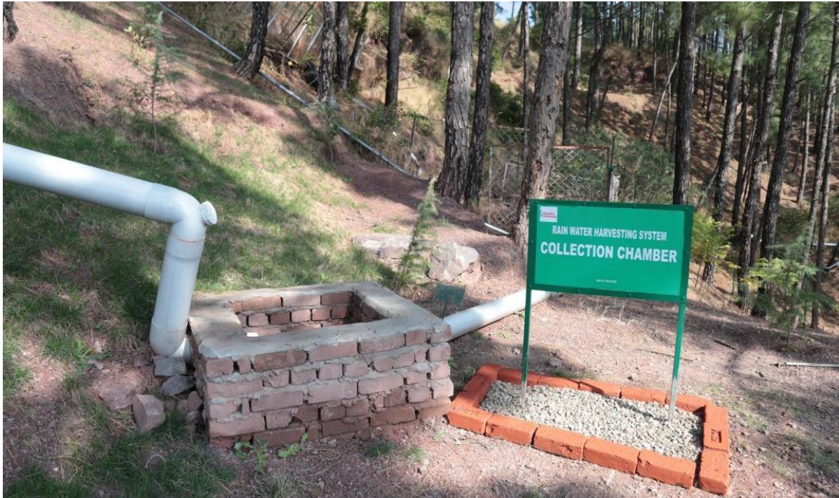
Figure 2: A rainwater collection chamber
